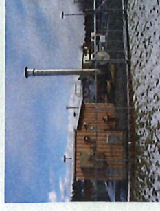
Metering and Regulating Station
